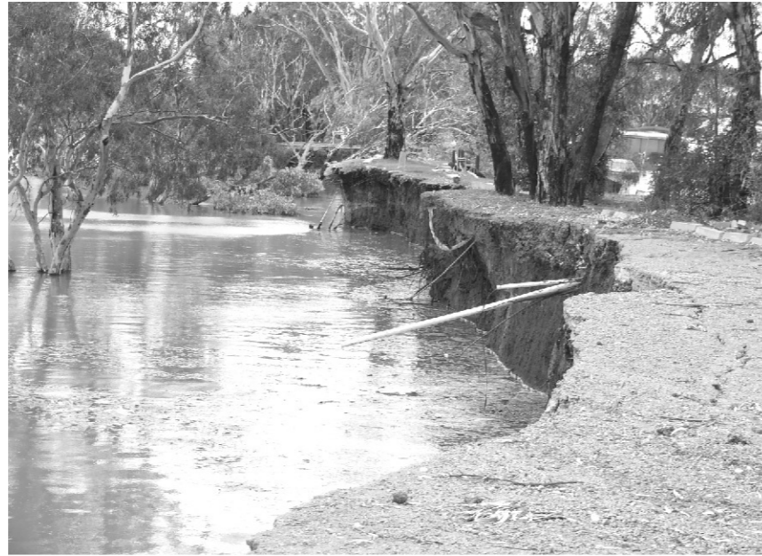
Slumping at Long Island Marina
